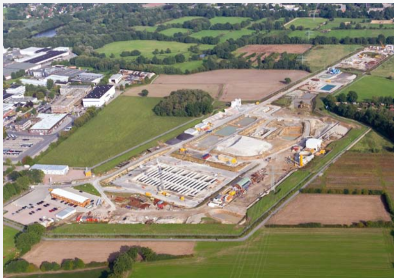
Figure 7 Left Simulation of the completed underground experiment hall and the above-ground laboratory and office building on the Schenefeld site Right Aerial view of the Schenefeld site (September 2010)
