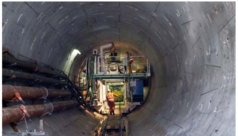
Figure 9 View of the first metres of the tunnel XTD1 with the end of the TBM in the back (July 2010)
