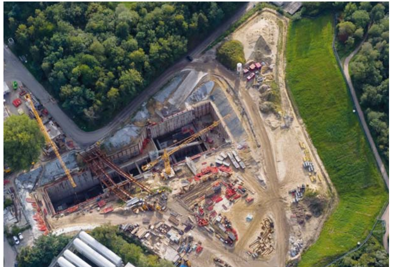
Figure 3 Aerial view of the injector complex region on the DESY campus (September 2010)
