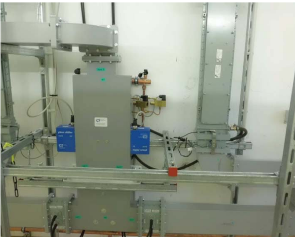
Fig. 7 5 MW power divider and 1 MW isolator in the AMTF shielding tunnel.
