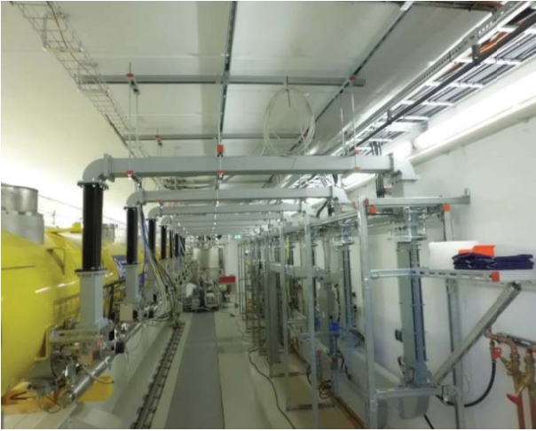
Fig. 6 Waveguide distribution connected to a cryomodule in the AMTF shielding tunnel.
