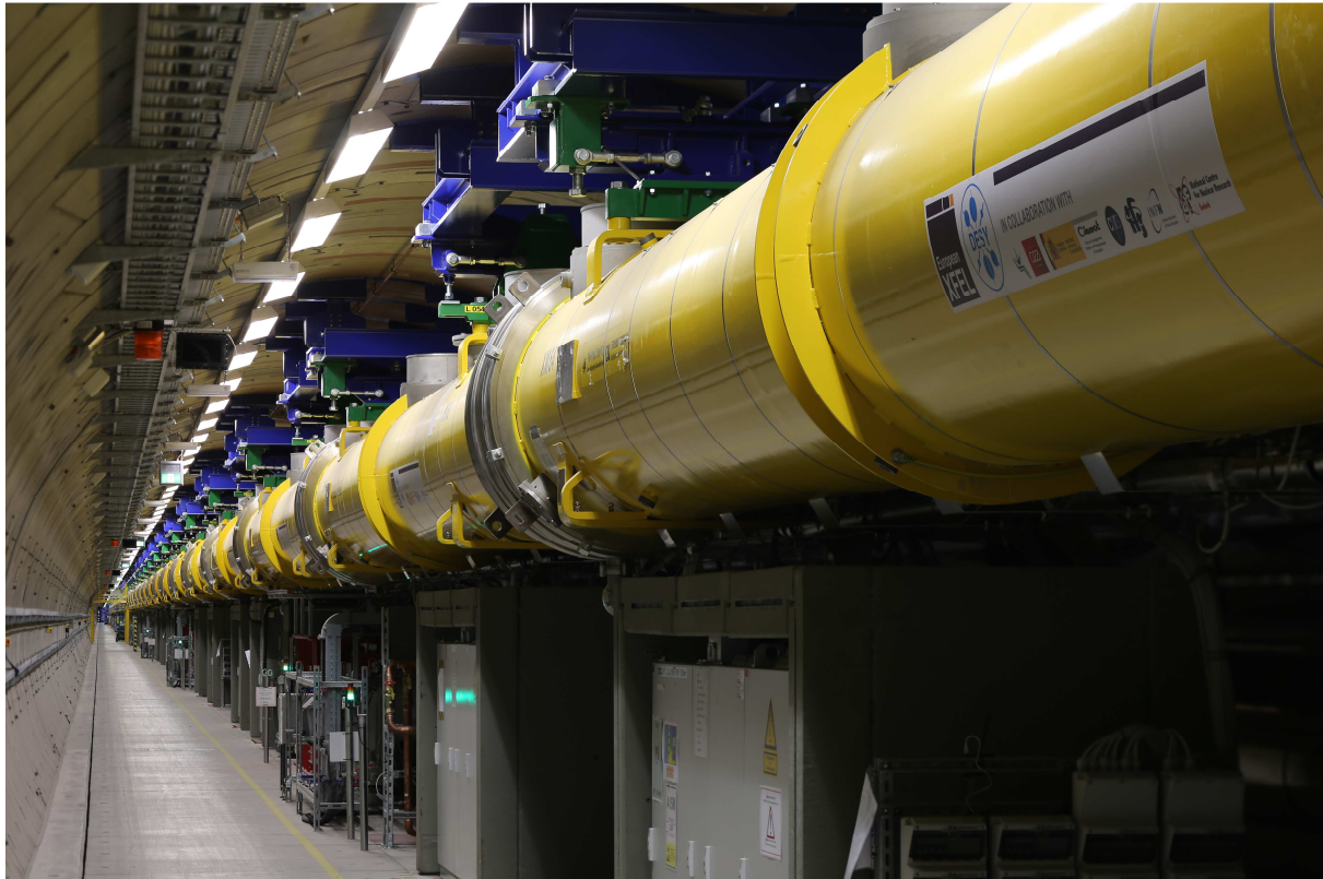
Figure 1. Completed main accelerator in one single tunnel. On top accelerator modules and cable trays. Below RF stations, electronic racks, power and water supply etc.
