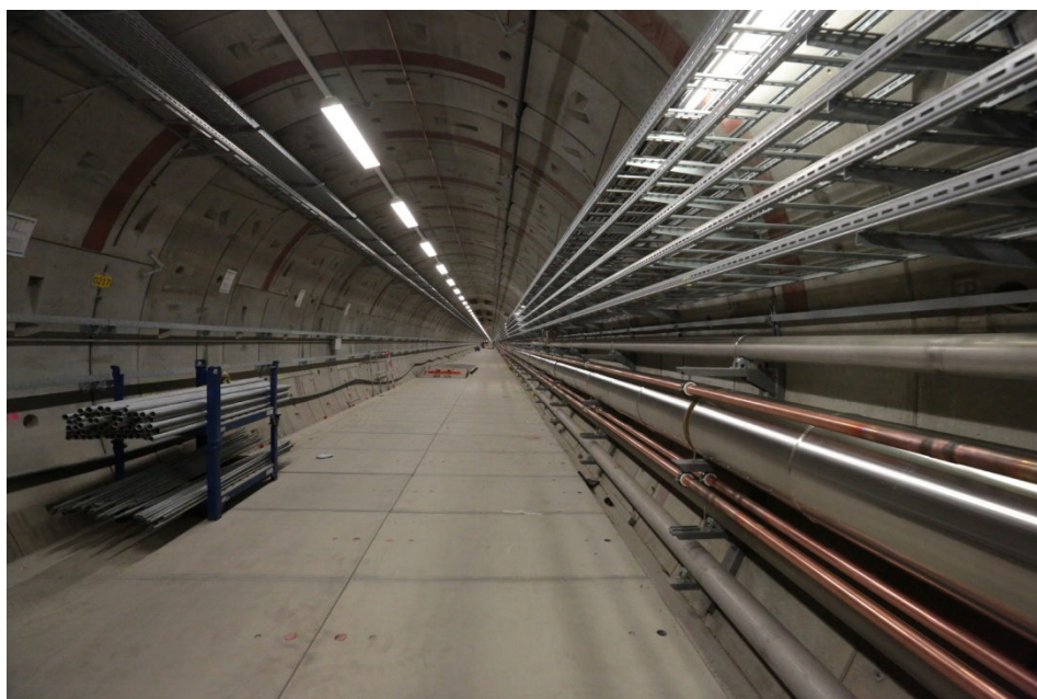
Utilities installed in accelerator tunnel
