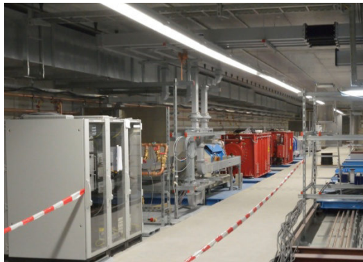
RF power components
