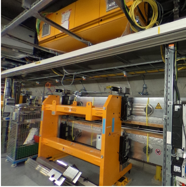
Figure 5.2: Picture of the exemplary undulator cell 32 of the SASE1 beamline during the construction phase. Credit: European XFEL GmbH
