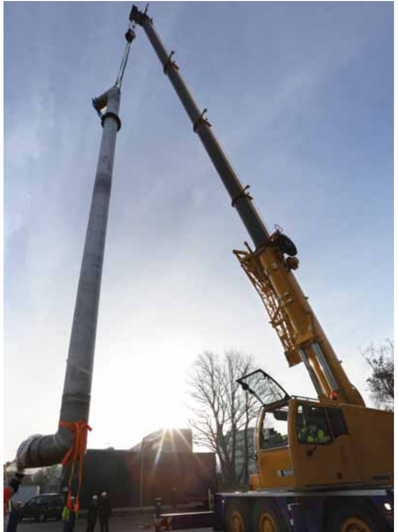
Figure 8 Another vertical cryogenic transfer line (February 2014)
