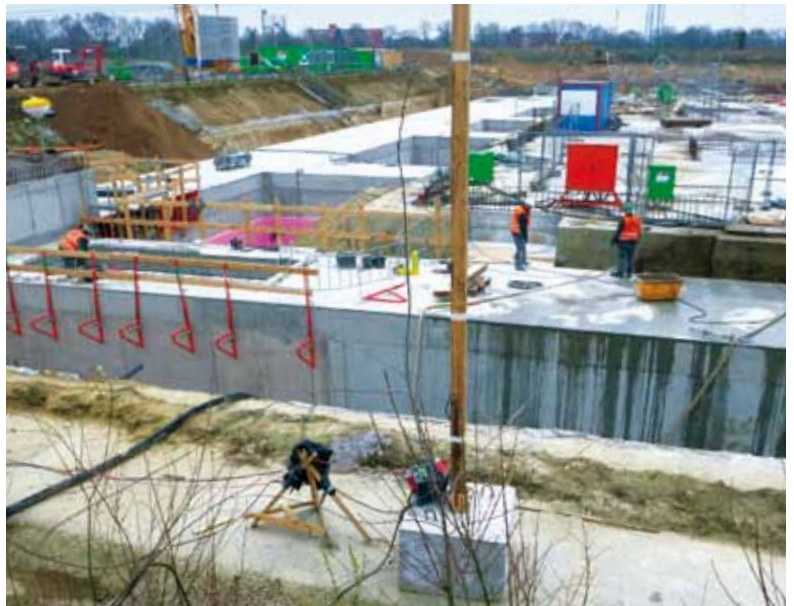
Figure 4 Completed media channels, located within the concrete structures, routed towards XHEXP1 on the Schenefeld campus (March 2014)
