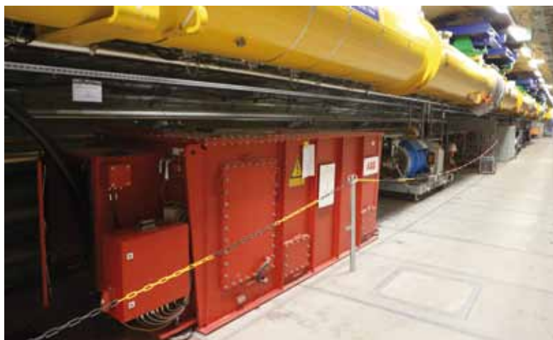
Figure 10 Installed accelerator modules in the L1 section
