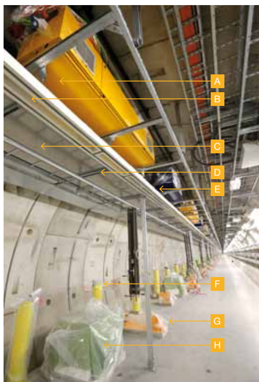
Figure 1 Status of SASE1 installation in the XTD2 tunnel in November 2014. Installed in the tunnel are undulator control racks (A), guide rails (B), enclosure and gasket seals (C), support frame (D), intersection control racks (E), vacuum posts (F), floor mounts (G), and concrete pillars (H).
