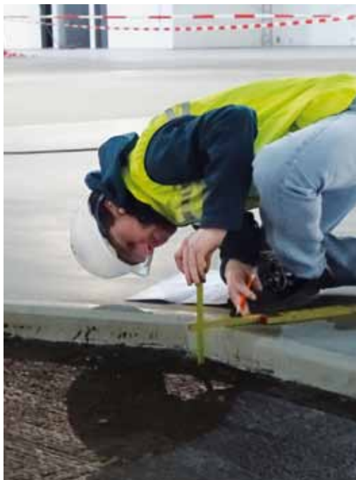
Figure 2 Inspection of the recess clearance for the SCS high-planarity floor after the casting of the main concrete floor in the experiment hall (XHEXP1)
