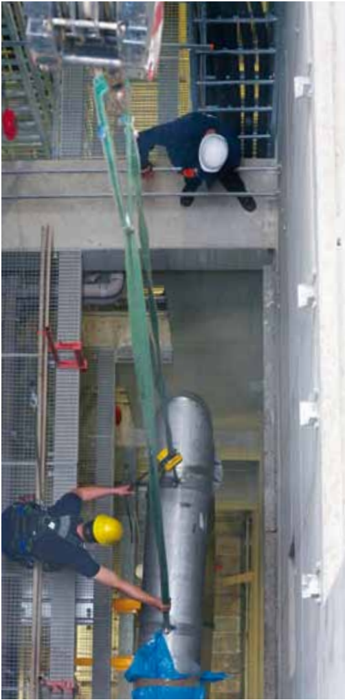
Figure 7 Inserting a vertical cryogenic transfer line into the media shaft in the entrance shaft XSE (May 2014)
