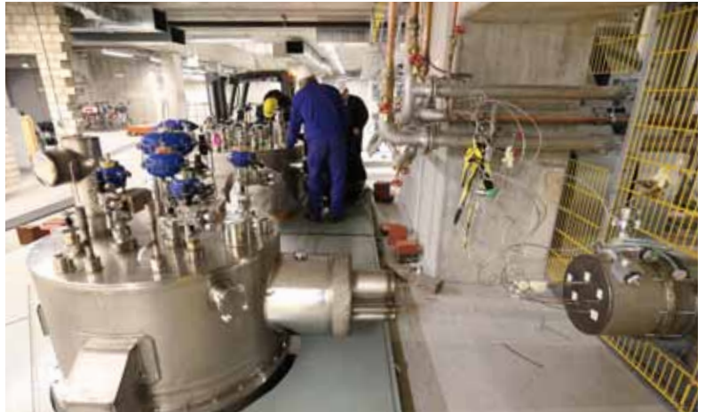
Figure 6 Installation of the cryo-valve boxes for the injector and linear accelerator cryogenic supply (November 2014)
