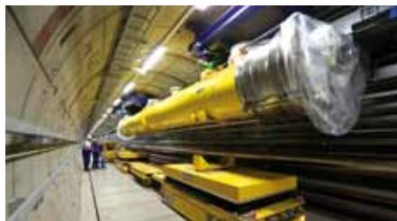
Figure 17 Installation of the first completed and tested accelerator module in the tunnel in August 2014
