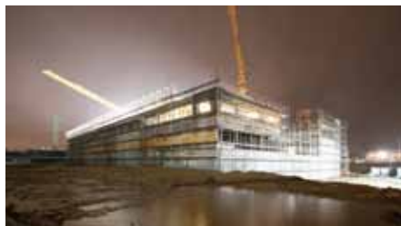
Figure 16 The European XFEL laboratory and office building (XHQ) under construction in December 2014
