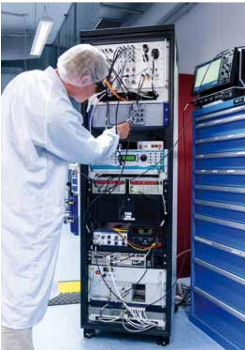
Figure 2 Control cabinet of the pump–probe laser
