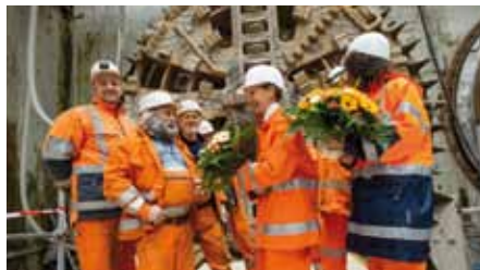
Figure 14 Arrival of the second tunnel boring machine in the final reception shaft on 4 June 2012
