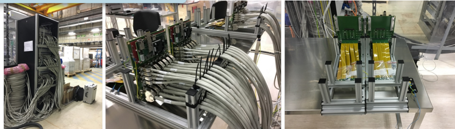
MPOD Crates with 29-m long Cables & Strain Relief
